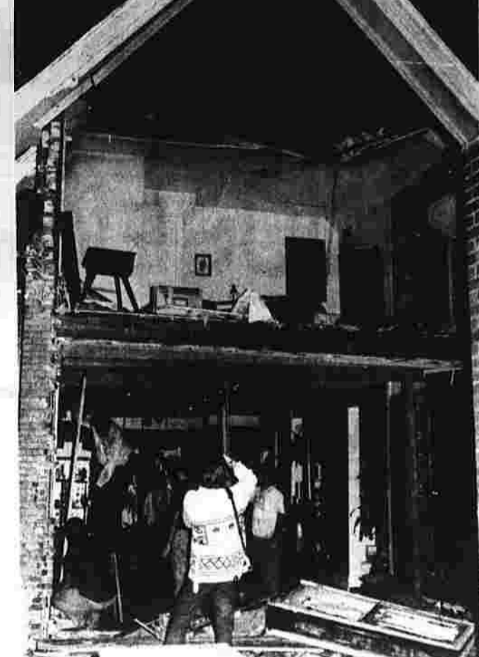
Shop Loses Wall
